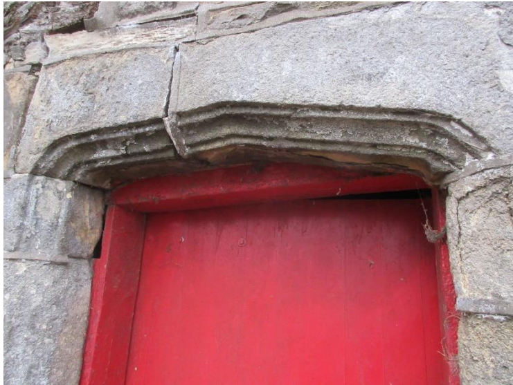
Reused early doorway in barn to the of the west of driveway
